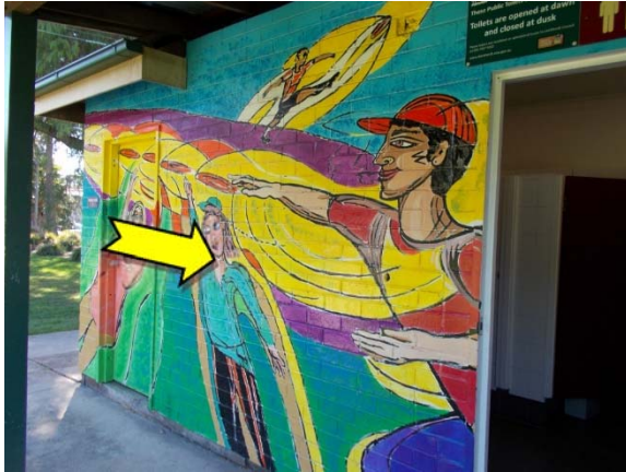
Photo 7. Exterior, throughout, graffiti walls – suspected lead-containing various upper coloured paint systems.
