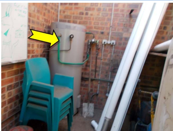
Photo 5. Interior, store room, hot water heater – suspected SMF internal insulation material.
