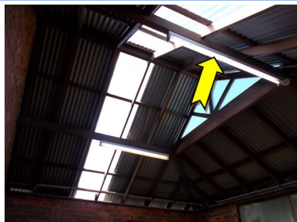
Photo 6. Interior, throughout, single tubed fluorescent light fitting – suspected PCB-containing capacitors.
