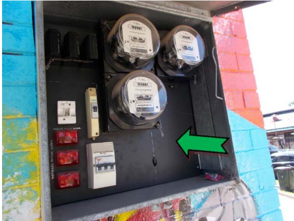
Photo 1. Exterior, south elevation, to wall, electrical board – suspected non asbestos-containing bituminous backing board
