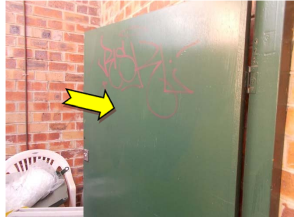
Photo 8. Interior, toilet cubicles – suspected lead-containing dark green upper paint system.
